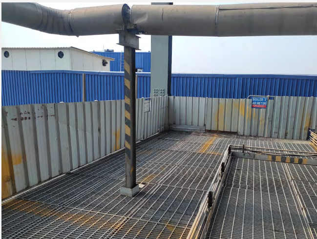
Cladding sheet barrier at height to prevent Gravitational Hazard
