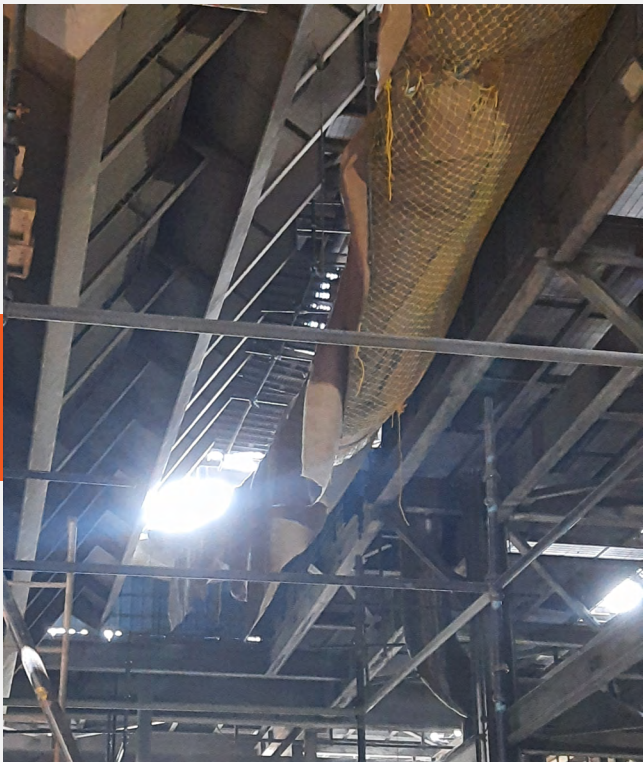
Use of Safety Net as Gravitational Hazard Control
