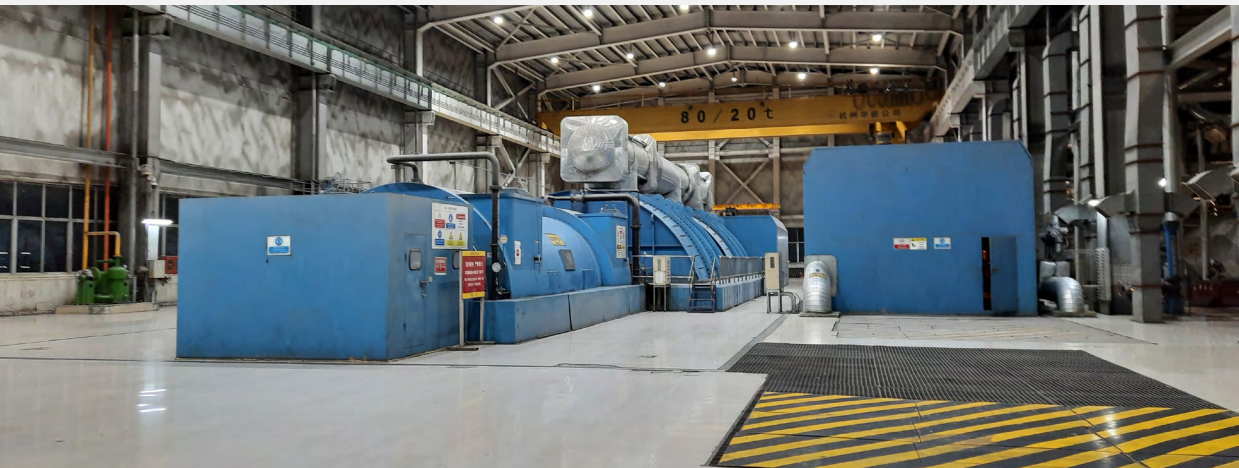
LED lights installed at Turbine floor of JPL
