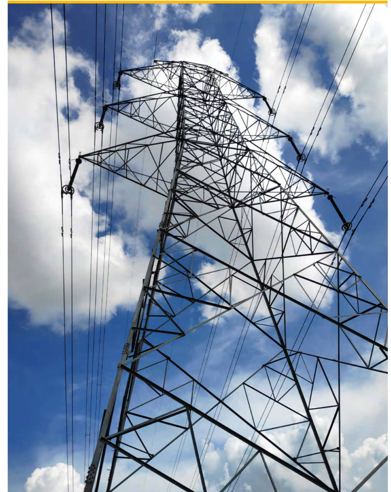
A Transmission Tower at Kohima-Mariani Transmission Line
