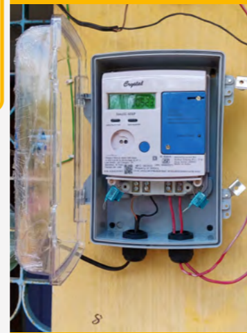
Smart Meter installed at Bongaigaon, Assam
